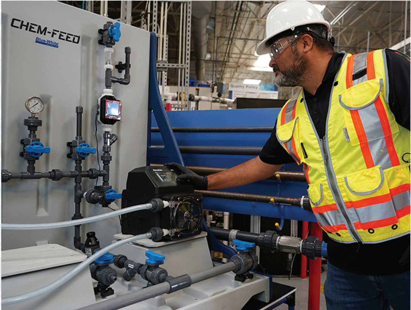
Testing of a CHEM-FEED Skid System
