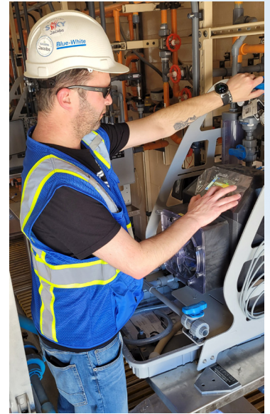
Figure 2. Peristaltic Pump Startup at a Water Treatment Plant.
